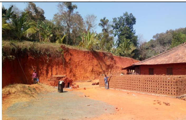
Photo 3: Extensive Cut Slope for making bricks & settlement, Vill. Chandrali, TS No. 48I/8.
