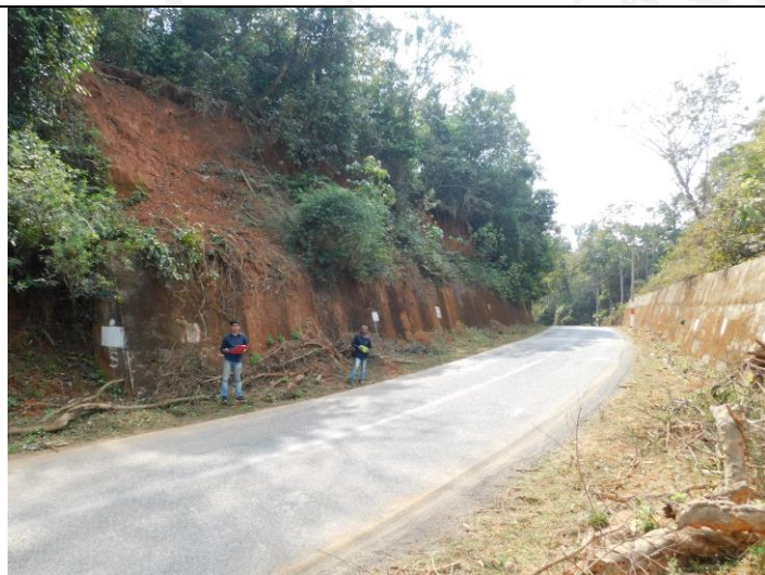
Photo 5: Slope failure with retaining wall on both the side of road, West of Vill. Ghotaki, TS No. 48I/8
