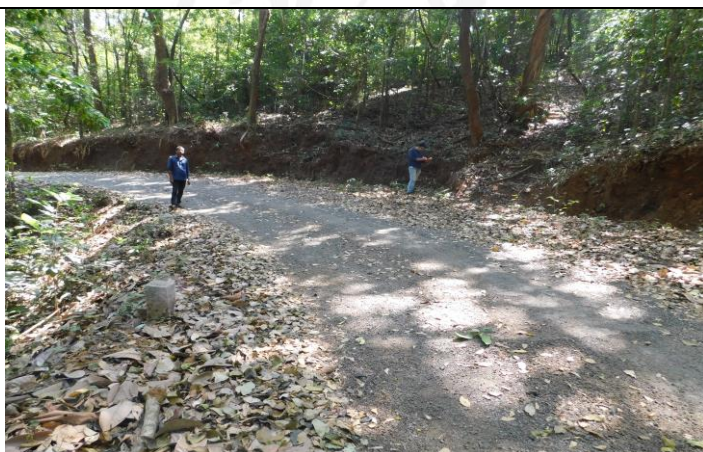
Photo 15: Natural course of nala obstructed, Road cracks observed due to removal of soil underneath indicating subsidence, SW of Kanangaon; TS No. 48I/8
