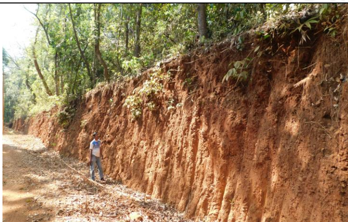
Photo 17: Extensive vertical cut slope observed in West of Kutvali; TS No. 48I/8.
